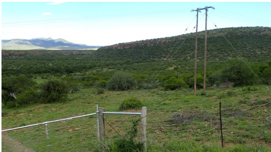
Figure 19: Photograph of existing power line along MR00639
